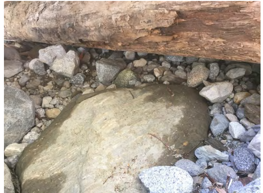
Right bank sill log scoured and only bearing downstream 2m length and 0.5m length at upstream wheel path location
