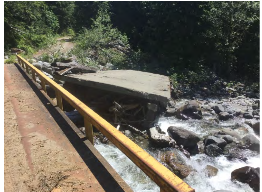
Old structure still remains in stream
