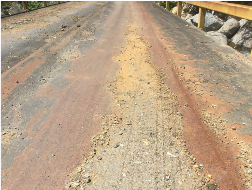
Steel deck plate deformation
